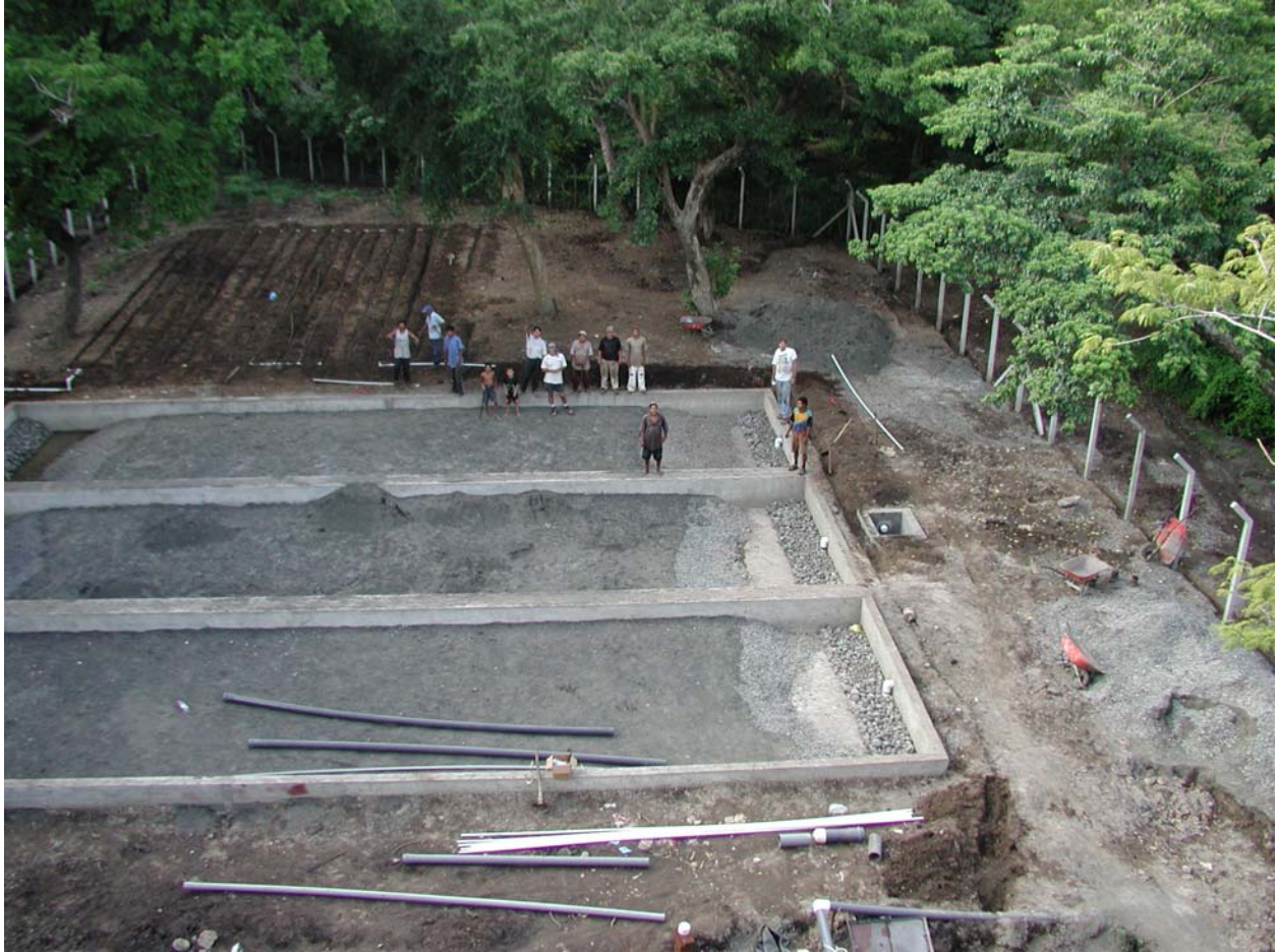
View of the Drip Field and Wetland Beds from High Up in a Tree
