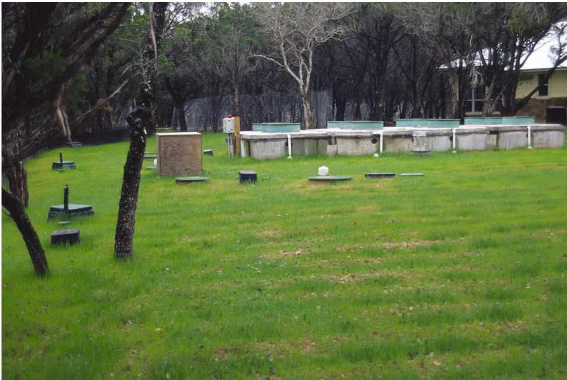
Treatment Center with Drip Field Surrounding It
