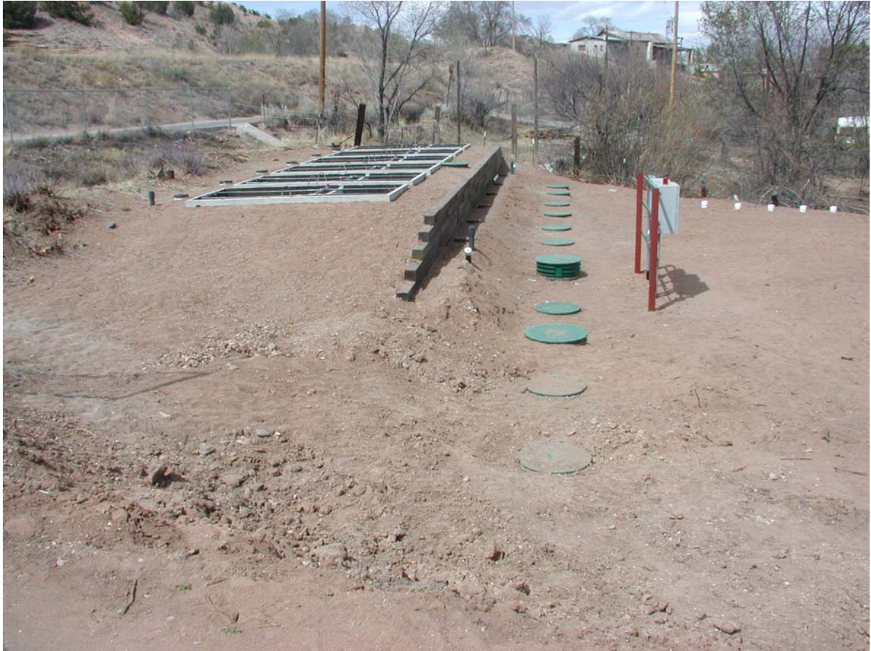
The Installed Treatment Center, Prior to Covers Being Installed on Filter Beds
